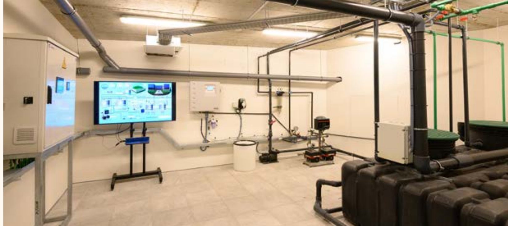
Interior of the underground hybrid wetland installed at the Las Tablas Corporate Headquarters (Madrid).
